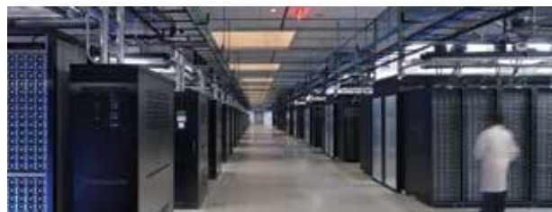
Server racks inside Facebook's 350,000 square foot Data Center
