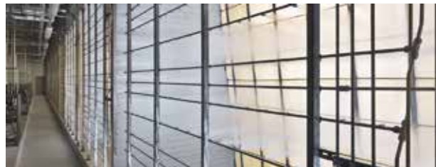
Misting fans help provide proper humidity level for outside cooling air
