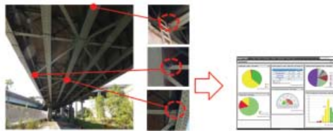
Sensors provide continuous information on the bridge condition. By identifying key locations the right information can be readily available to all decision makers via interactive web interfaces.
