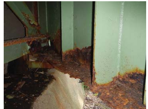
Severely Corroded Steel Girder. Corrosion Caused Primarily by Leaking Expansion Joints
