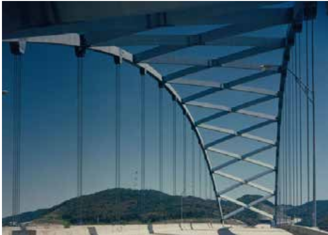
I-470 Tied Arch over the Ohio River, Wheeling, WV Photo Courtesy of HDR, Inc.
