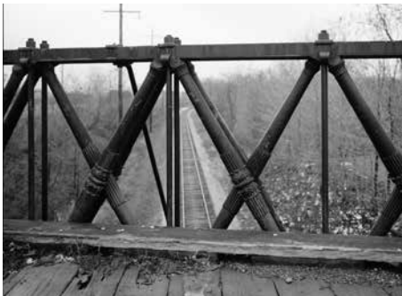
The Reading-Halls Station Bridge (1846), U.S. Route 220, spanning railroad near Halls Station, Muncy, Lycoming County, PA, is almost certainly the oldest all-metal (Howe) truss bridge in active service in the United States, a lone survivor from the first series of all-metal trusses of any kind designed and constructed in the United States. A characteristic of the Howe truss is the introduction of internal prestressing in the diagonals through tensile forces applied to the vertical members during fit-up at erection.
