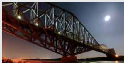
Quebec Bridge, spanning the St. Lawrence River, Quebec, Canada (photo courtesy of WikiCommons)
