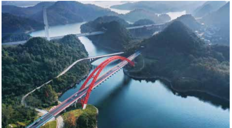
Huayudong Bridge Removal and Reconstruction Project; Shanghai-Kunming State Highway (G320) Guiyang Section, Guiyang, Guizhou, Peoples Republic of China
