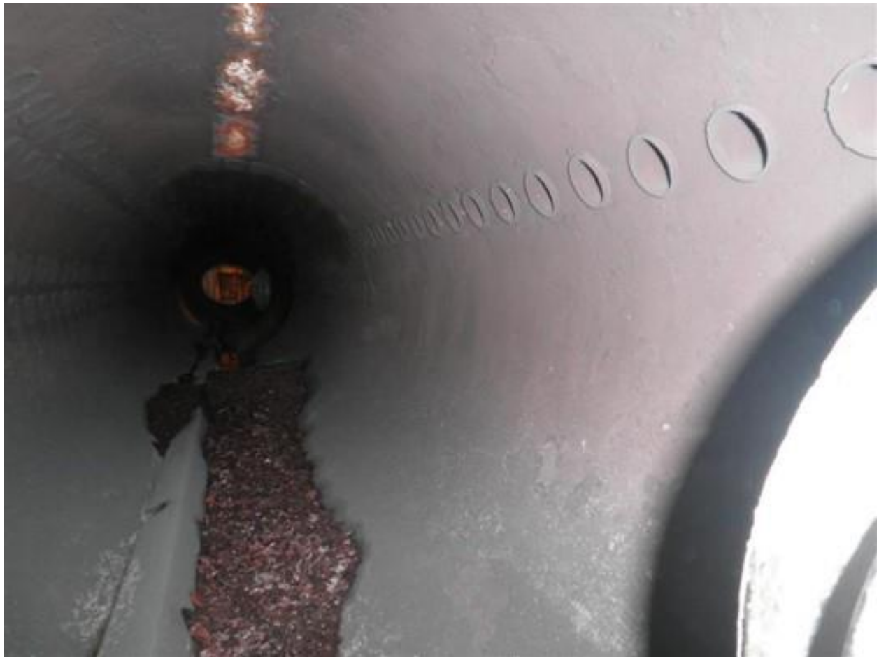
Figure 3: Boiler mudrum with carryunder, but no tubes present near steam blanketing.
