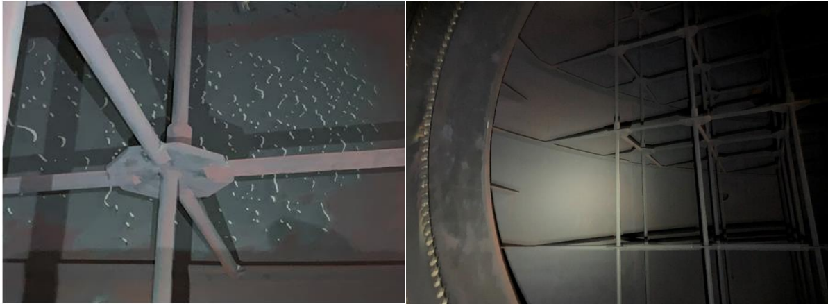
Figures 11 and 12. Tiger stripe pattern in turbine exhaust duct hotbox area indicating two-phase FAC prior to FFA treatment (left). 10 months after FFA treatment, two-phase FAC pattern is absent (right).
