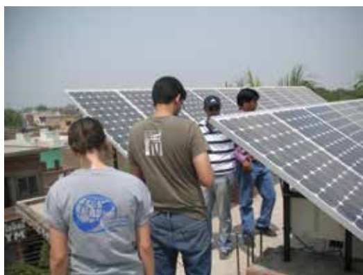
EWB Travel Team members inspecting completed photovoltaic system on Symbiosis Public School in Rampur, India
