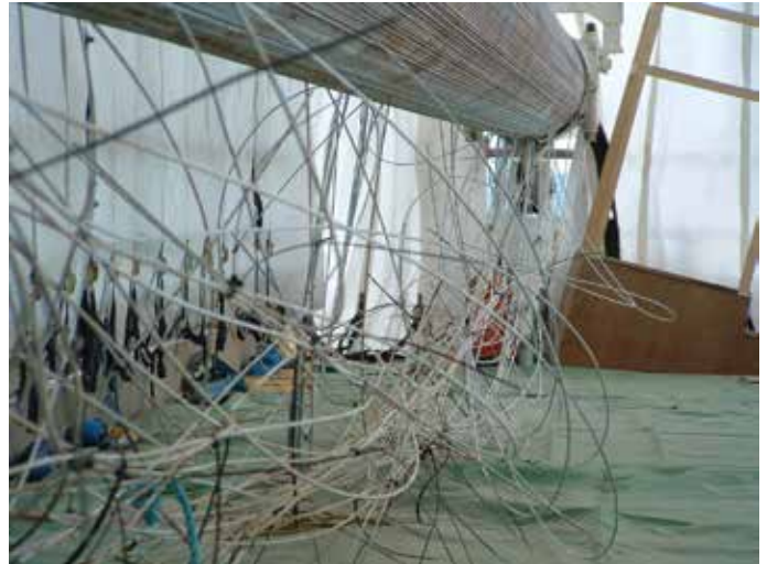
Figure 3 Cable Wire Breaks (Photo courtesy of AECOM)
